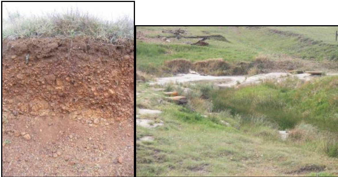
FIGURE 6: DOLERITE (LEFT) AND SANDSTONE (RIGHT) ARE THE TWO MAIN GEOLOGIES FOUND ON SITE
